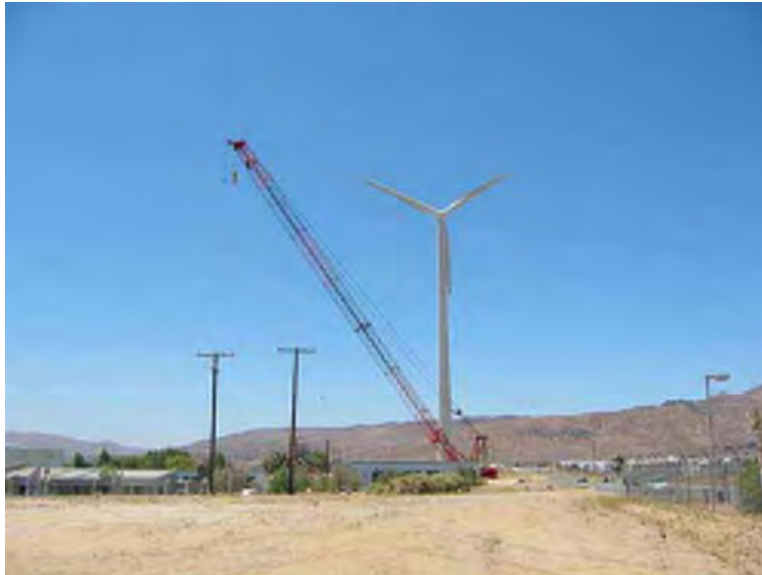
Figure 7 Wind Turbine and Crane
