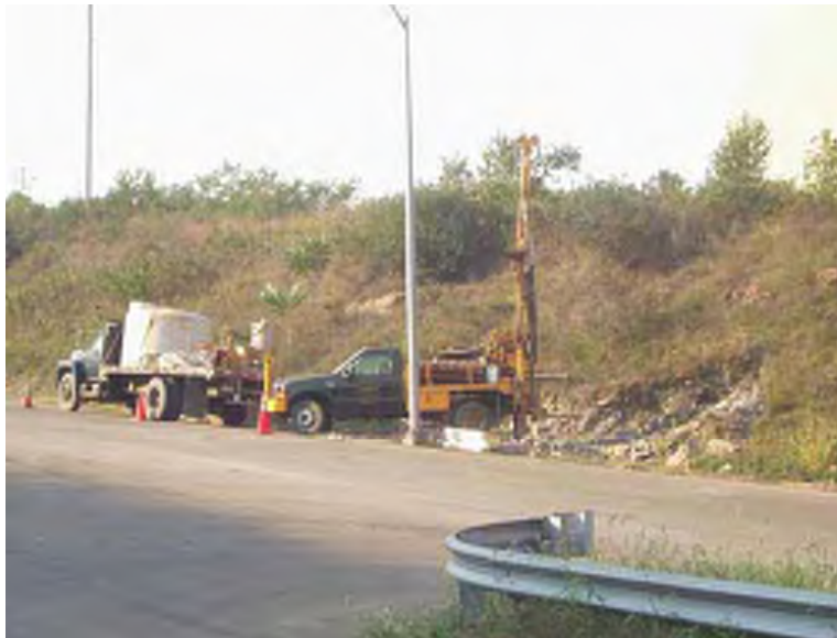
Figure 12 Typical Coring Truck and Support Vehicle
